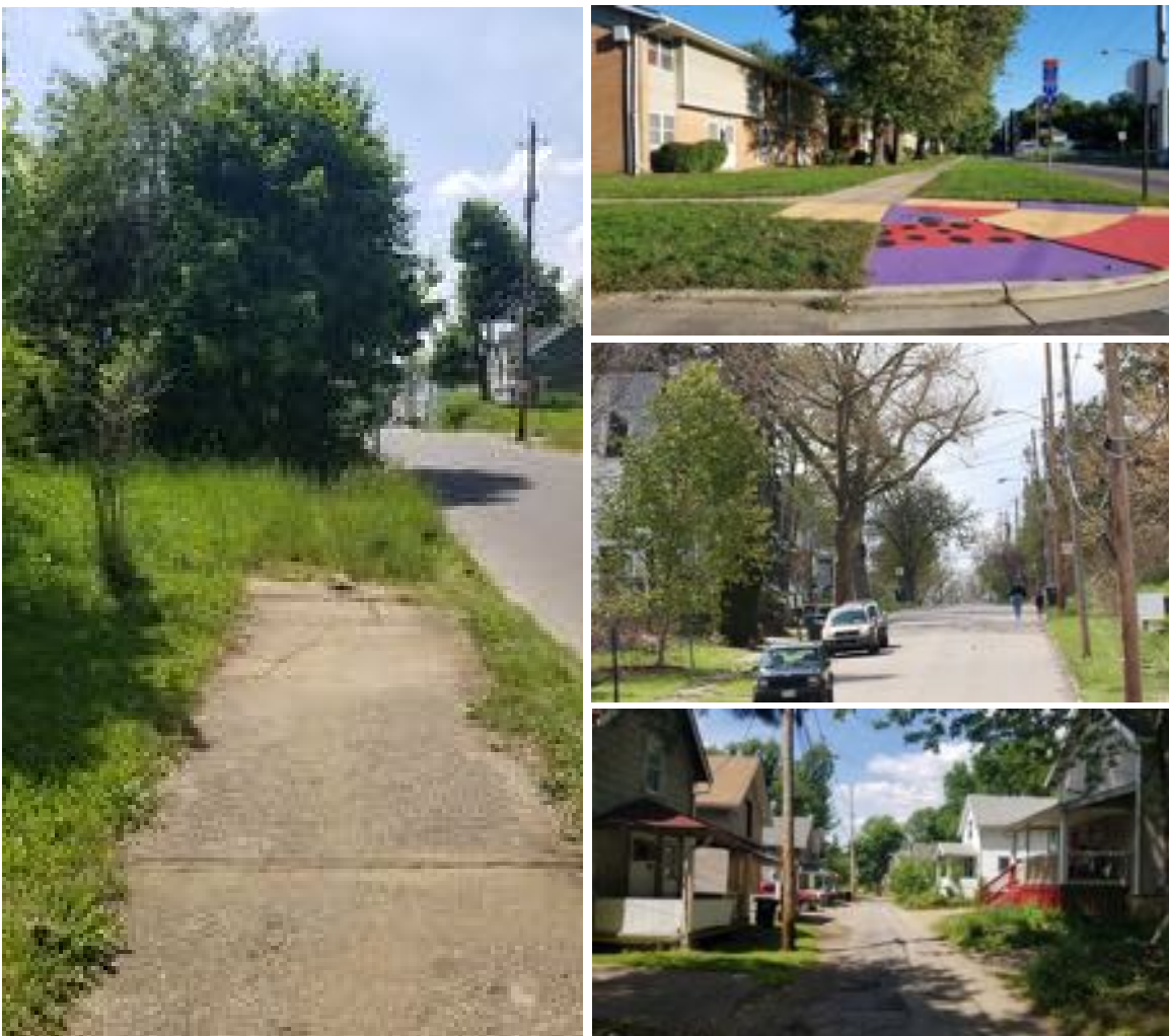
Examples of sidewalk conditions.
